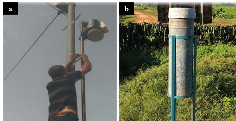
Figure 2. Illustrate the installation of automatic station (a) and rain gauges (b) for the purpose of monitoring climatic variables. Source. Photograph taken by the first author.
